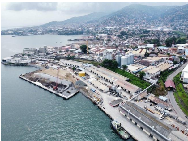
Figure 12 Drone photo (EGCM). New berth approaching completion in December 2023, showing crawler crane installing stone columns. Fenders and bollards in place.
