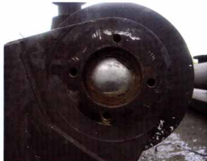
Figure 3: Inside a PM bottom bearing after two years in service
