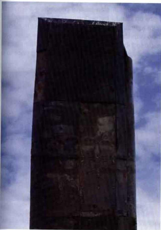
Figure 4: Loss of facings due to failure of fixing stud welds
