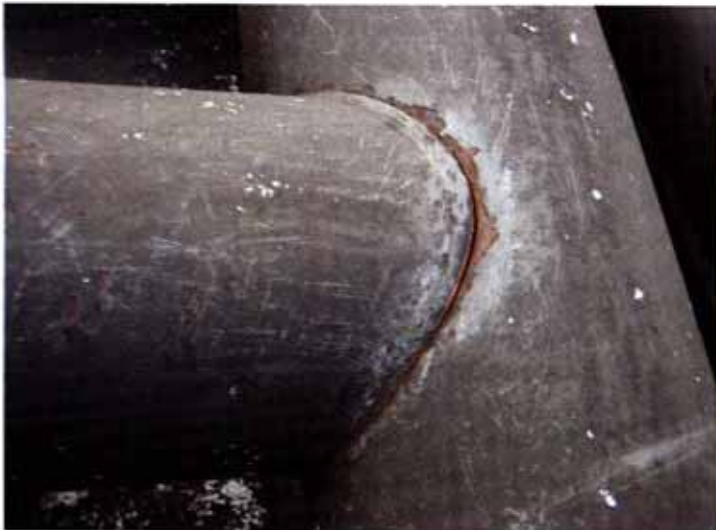
Figure 2: A torsion arm to torsion tube joint with cracked weld
